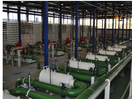
Alicante I Desalination Plant (Spain)
