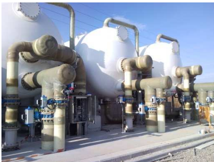
Delta de la Tordera Desalination Plant (Spain)
