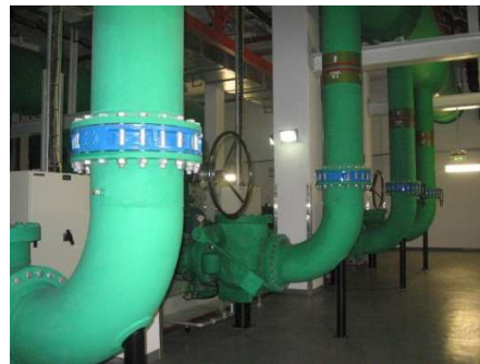
Burj Khalifa District Cooling DCP3 (Dubai)
