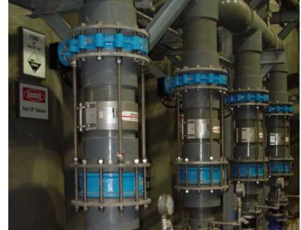
Ulu Pandan NeWater plant (Singapore)
